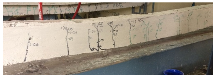
Fig 6: Crack pattern in HC rectangular beam
