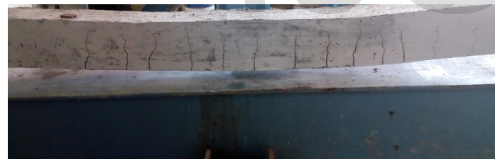
Fig 5: Crack pattern in HSC rectangular beam
